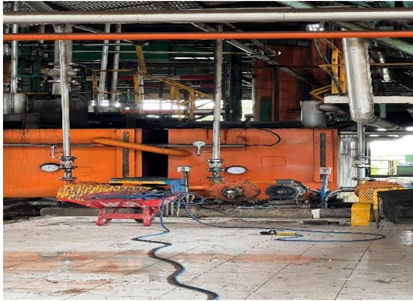
Gambar 4.1 Lantai Licin akibat kebocoran pipa
