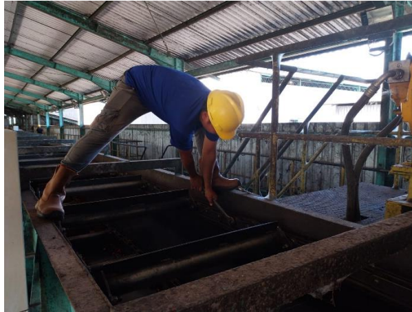
Gambar 1. Mekanik Preventive Baut Chain Screper Conveyor No 2
