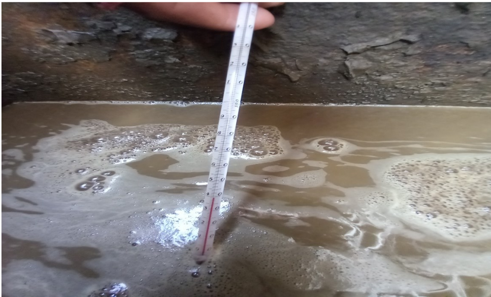
Pengukuran suhu coling tower
