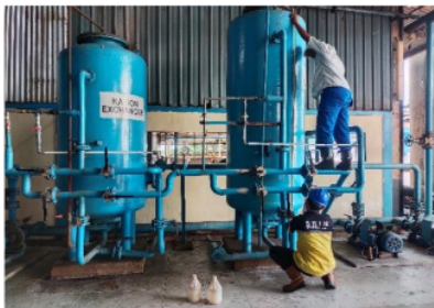
Gambar 3 Unit Demint Plant
