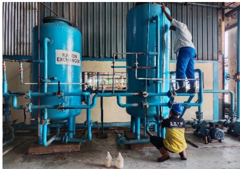
Gambar 3 Unit Demint Plant
