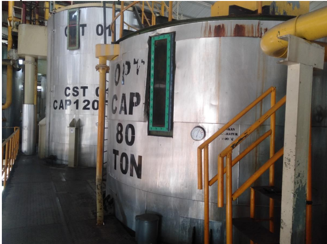
Lampiran 3. Gambar Oil Purifier Tank
