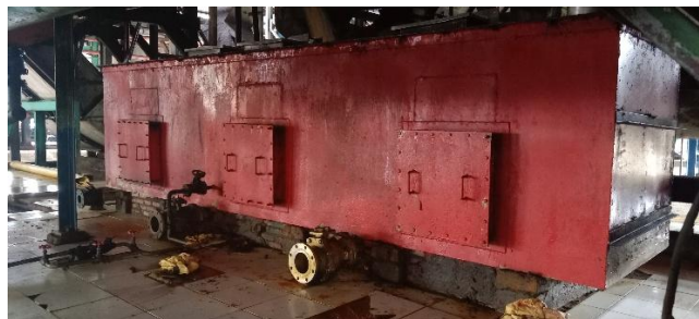
Gambar 3. 3 Crude Oil Tank
