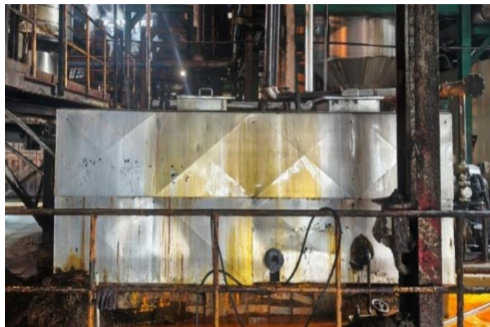
Gambar 1. Crude oil tank (COT)
